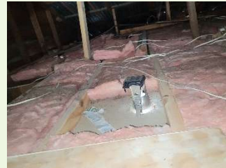
Old light fittings, gaps in insulation and direct path for heat to escape into the ceiling
