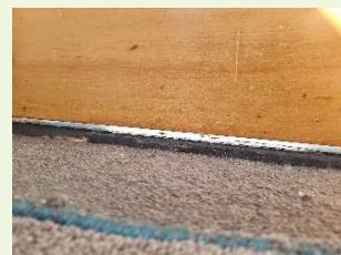
Gaps around doors and windows are a large source of heat loss in insulated homes
