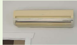
The old inefficient living room heat pump
