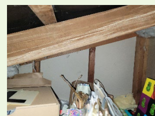
Wall insulation missing in ceiling space walls
