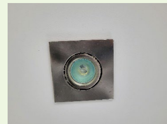
Halogen light fittings, gaps in insulation and energy wasted through excess heat created
