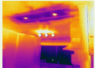
Before: Gaps in insulation around lights (dark colour = heat loss)
